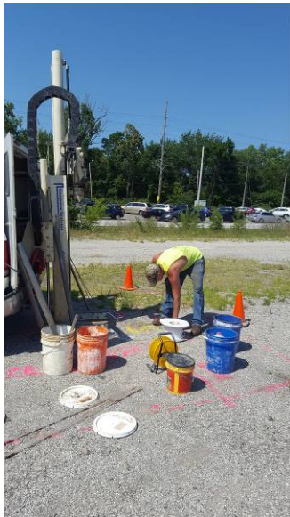
Photograph 3. A&W preparing to pump groundwater for a grab sample at Boring B-1-3-1, view to the north
