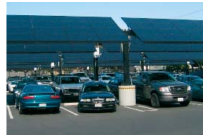
Solar panels utilized in parking lots can both generate electricity and provide shading for cars.
